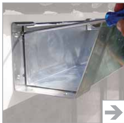
7. Anchor each joint union to the fascia board using 32mm x No10 screws, SC202. All angles should also be anchored in the same way.
